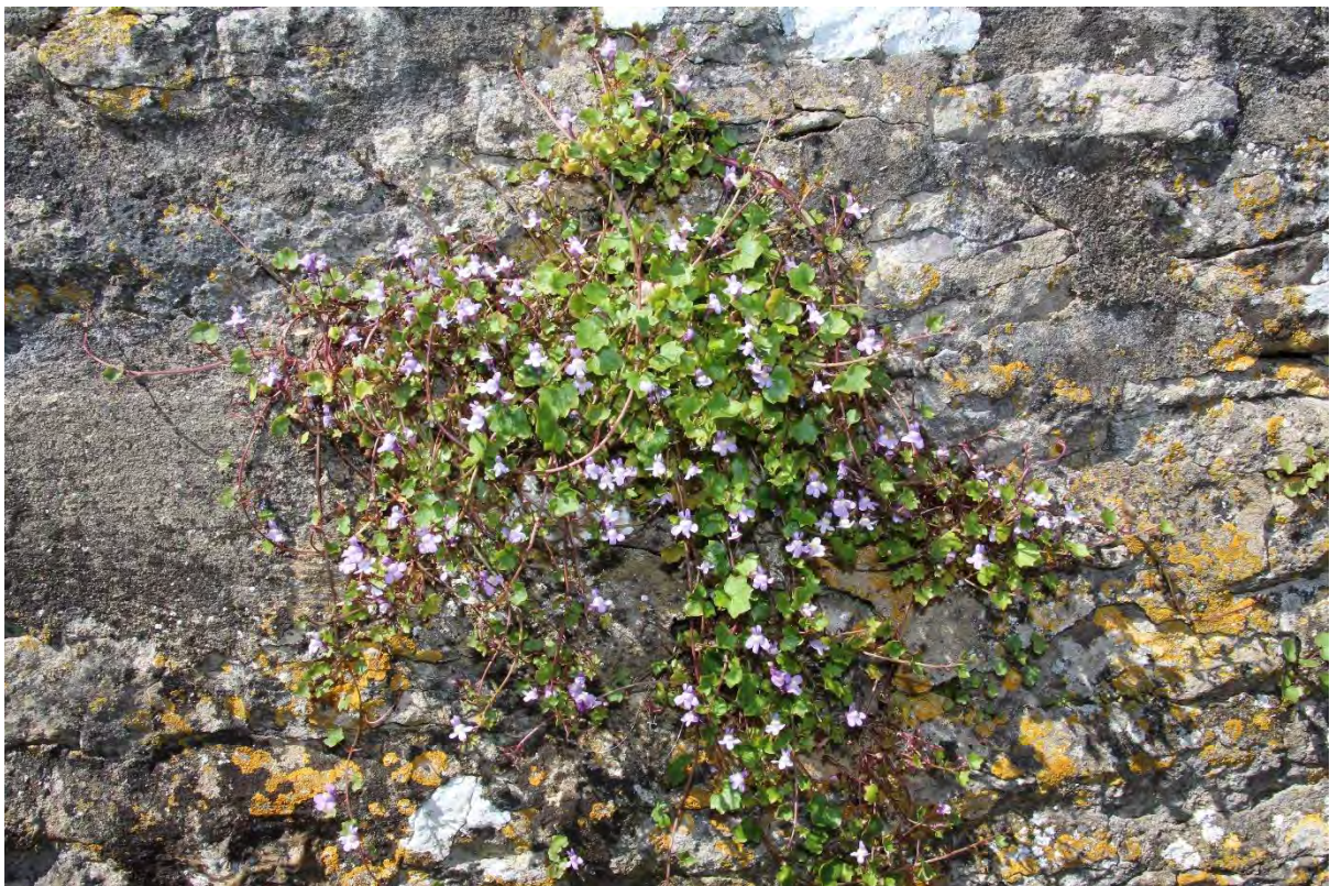
Figure 26. Kenilworth ivy growing on a much-repaired drystone wall on the Upper Green – Lower Green foot path. Note also the various species of lichens growing on the stone.
